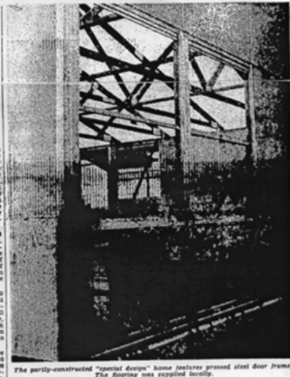
The partly-constructed "special design" home features pressed steel four frames. The flooring was supplied locally.
