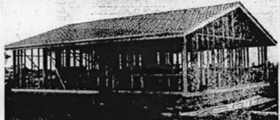
One of the ten conventional-type homes under construction at East Bairnsdale features locally supplied materials.
